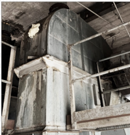
Existing Gear Unit - Foote Jones
